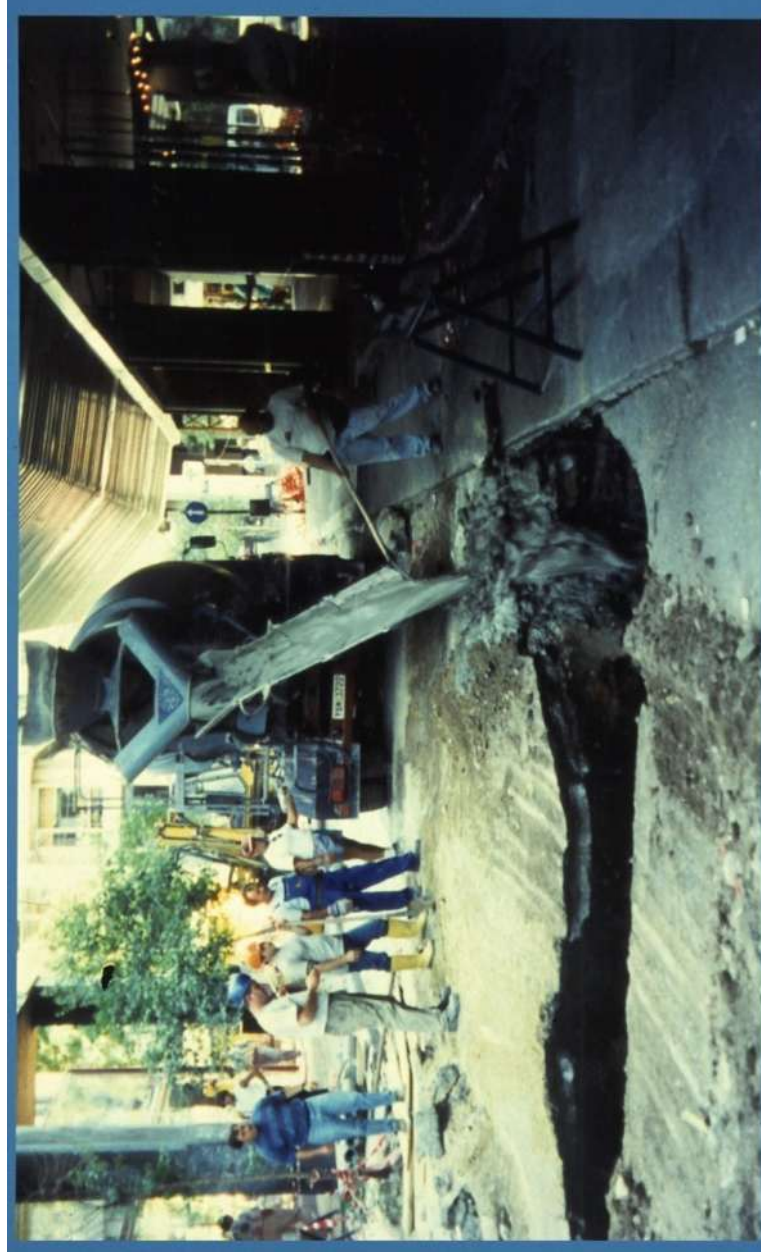
Collapse to surface above TBM drive at Nikis St.
