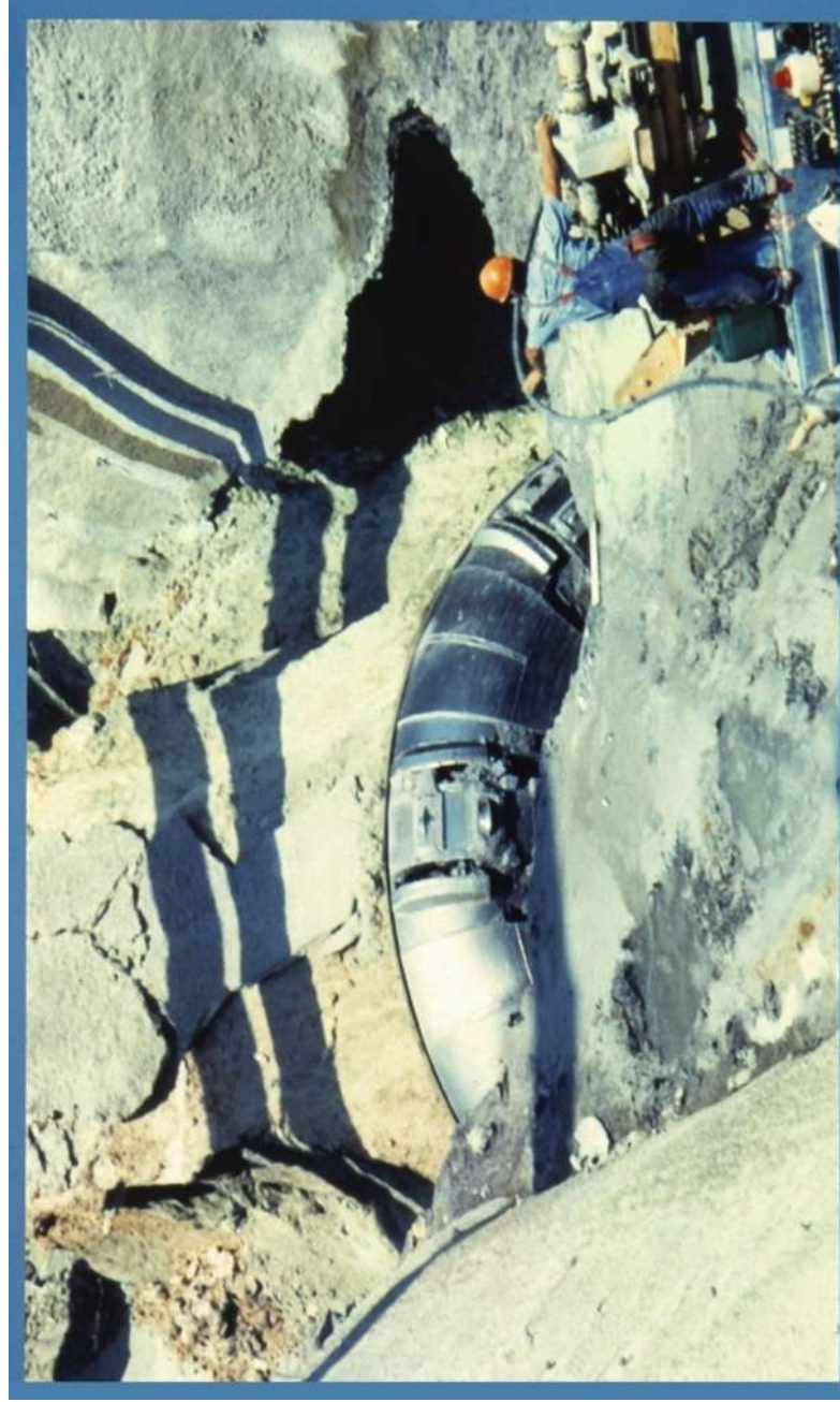
Collapse to surface above TBM drive at Karaiskaki Sq.
